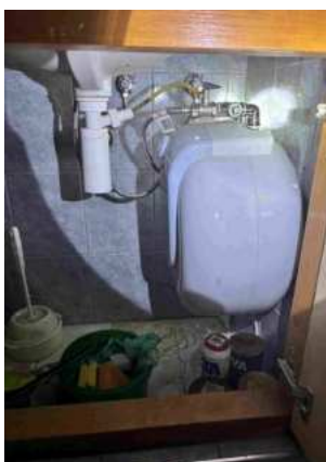
1.NP – el. boiler
